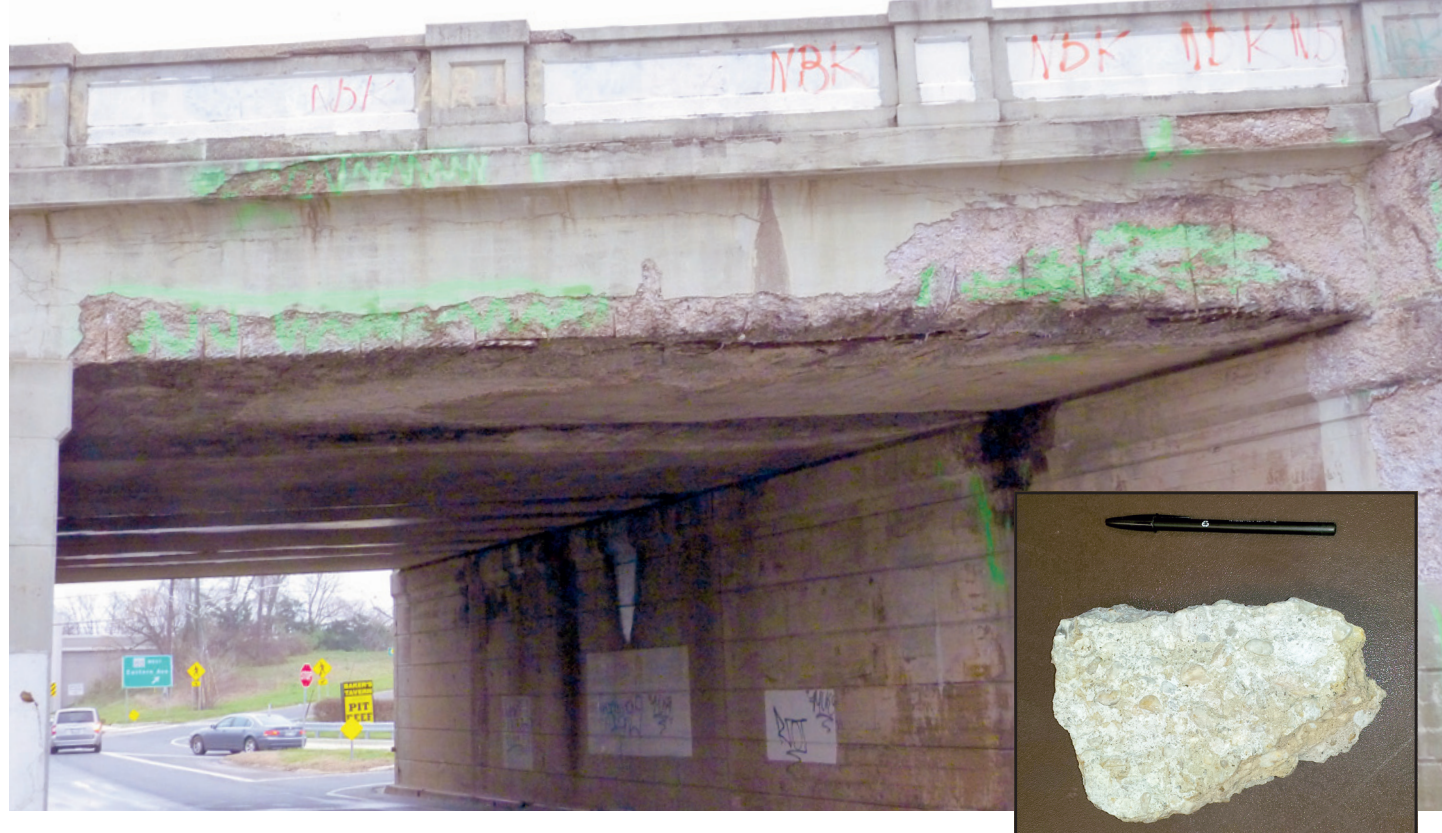
The deteriorating condition of this train bridge over Martin Boulevard in Middle River has become an increasing concern for drivers passing under it. Inset: A large chunk of concrete was found on the roadway of Martin Boulevard, having fallen from the ceiling above.
