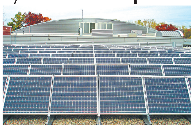
Maplewood Community Center’s solar panel system will be dismantled and stored. Ten K Solar, the Bloomington-based company that manufactured the solar panels for the project, recently declared bankruptcy.
