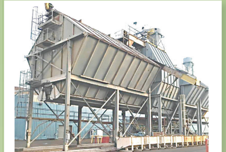
Two 30-Unit Chip Bins, 10392
