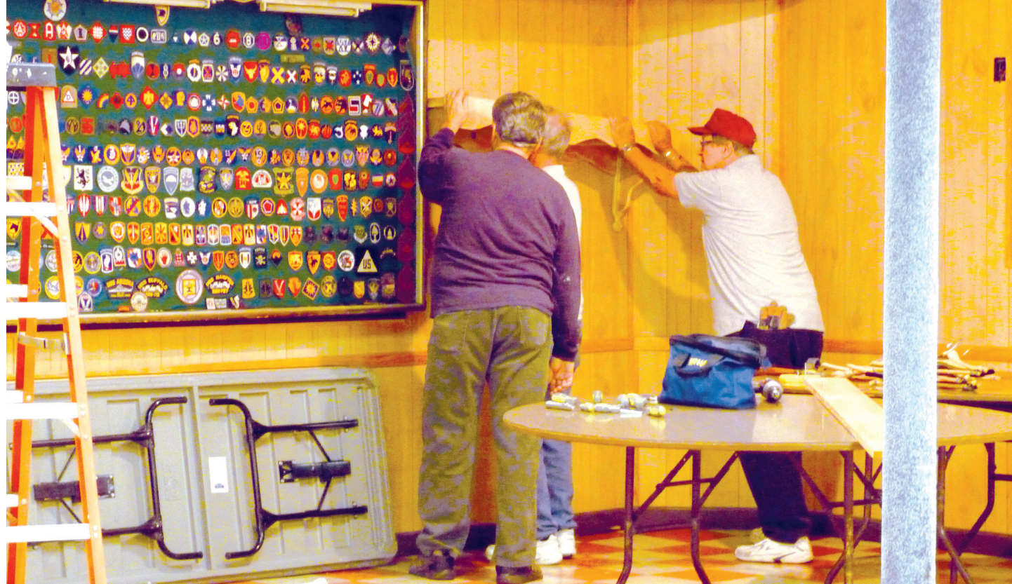
Charles Eving VFW Post 6506 members work to remove a shelf from a wall in preparation for the arrival of volunteers from The Home Depot, who spent the day on Oct. 28 renovating the halls, restrooms and roof of the largest VFW post in Maryland.
