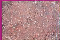
Both Cambridge paving stones shown were installed in residential driveways in 2006 (Photos taken in January 2010).
