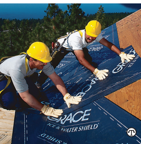
Using the proper roofing underlayment to repair damaged roofs also prevents future leaks.
