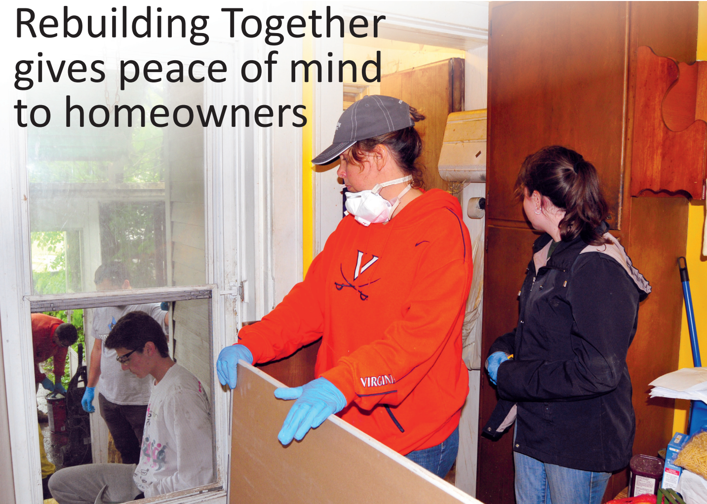
Inside John Kaiser's home on Dunbar Road, Rebuilding Together volunteers prepare to install a new section of ceiling while outside, other volunteers replace a porch landing.
