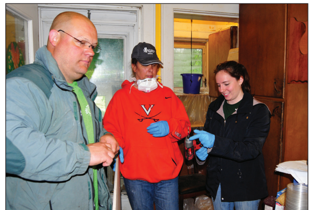
Improvement Zone owner Nick Neboshynsky (left), Leigh Ann Rawlins and Julianna Makarsky prepare to install a piece of new ceiling drywall.
