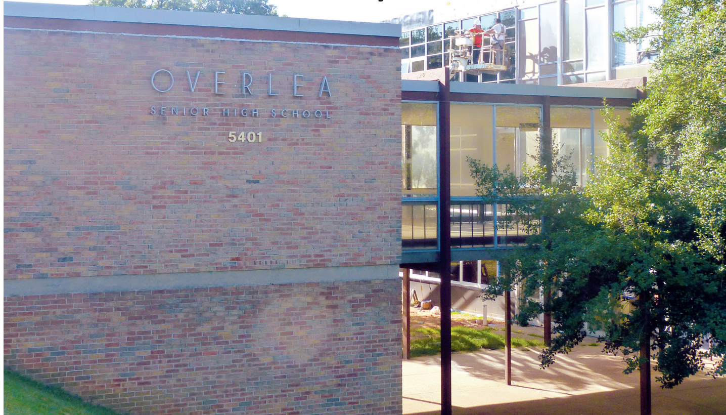
Workers install new windows on the front façade of Overlea High School as part of a two-year renovation plan that will replace all the windows in the school, add air conditioning and update classroom space.
