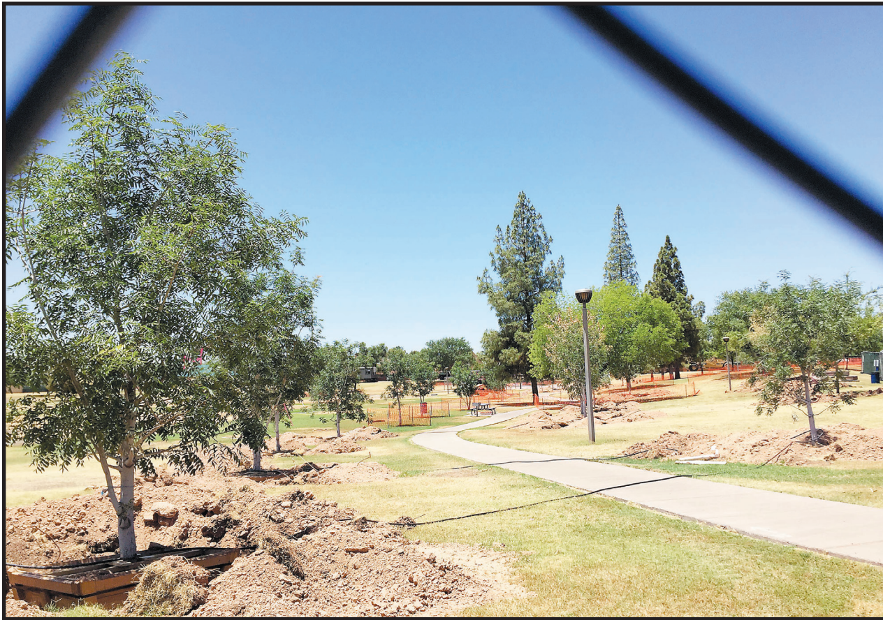
The chain-link fence surrounding Estrada Park near Warner Road and McClintock Drive was draped in tarp as construction work begins on a new fire station for South Tempe. Select trees, like the one pictured above, are being dug up and boxed for replanting in the park area. For more park construction photos see our Facebook page.
